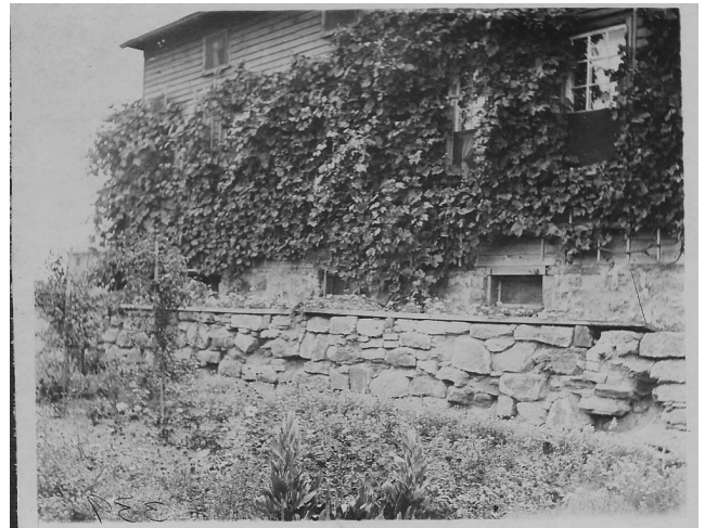
Above-grade basement windows. The rabbatt surrounding the building comes to the bottom of the windows.
